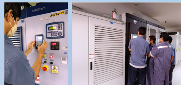
Reducing the Lower Speed Limit of Water Pumps from 70 percent to 50 percent
